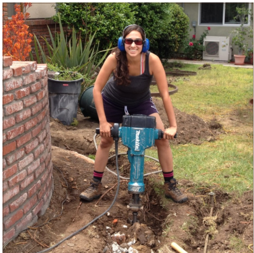
OH alumna Sara Bendrick wields a jackhammer on the job as host of the DIY network series “I Hate My Yard.”
